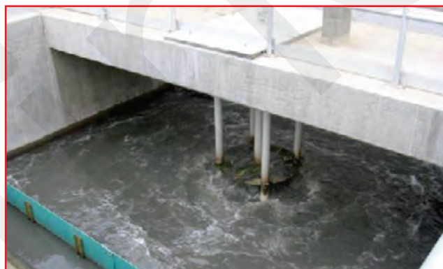
Grit and sand removal tank
